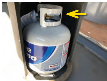
Find valve at top of tank
